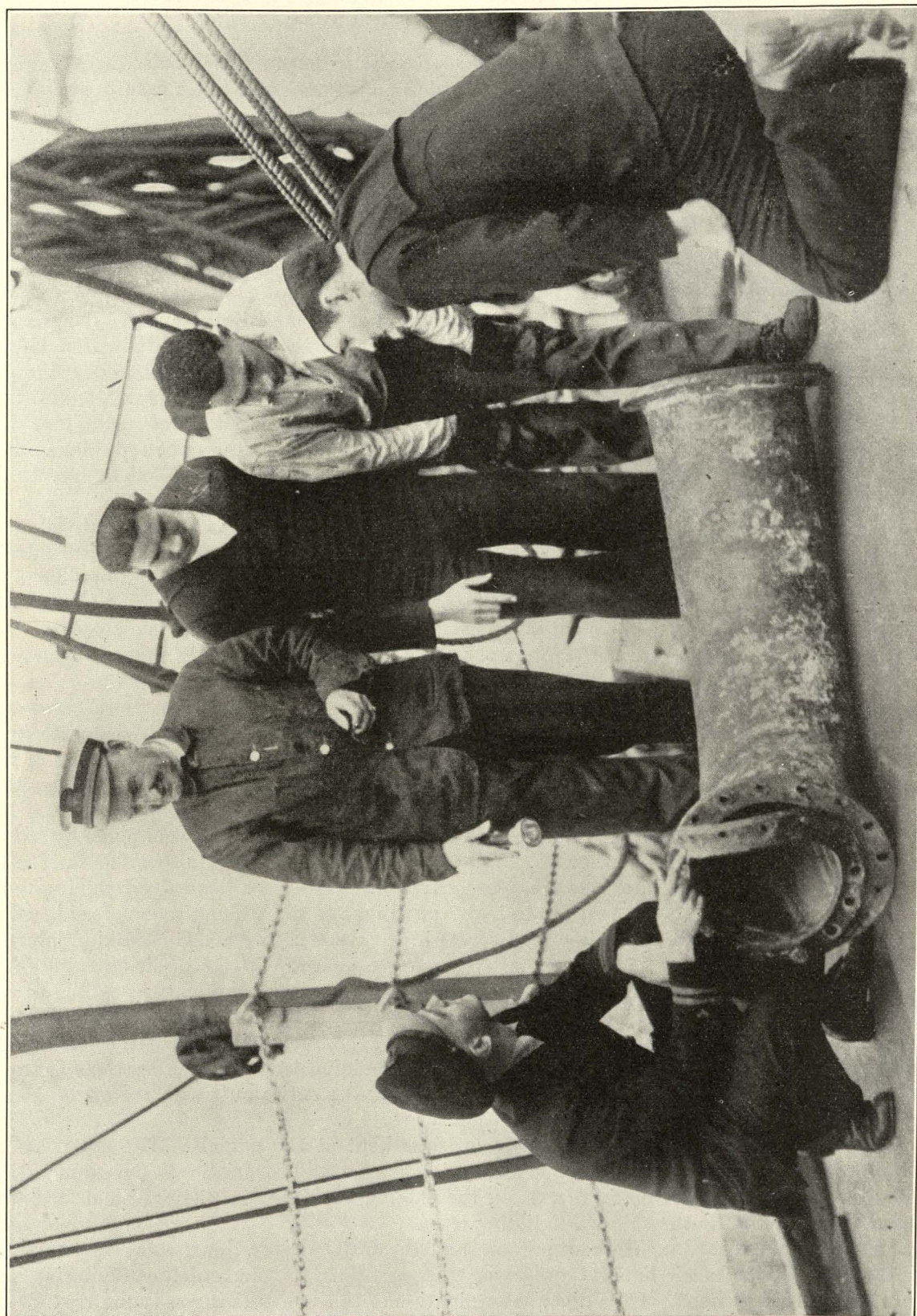
FIG. 10.—SECTION OF 12-INCH AIR SUPPLY LINE TO MOTOR ROOM, REMOVED BY DIVERS
