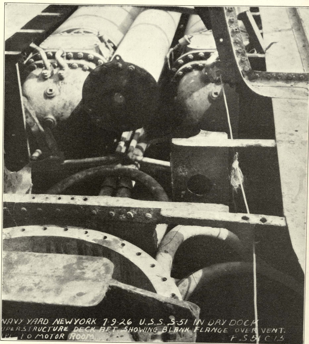
FIG. 11.—TWELVE-INCH SUPPLY PIPE TO MOTOR ROOM SEALED BY COVER PLATE INSTALLED BY DIVERS
